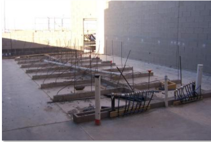
Photo above shows poor protection of vertical steel.
