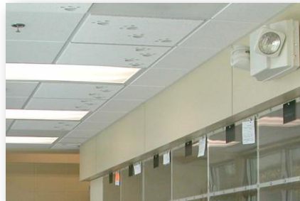
Paw print, acoustic lay-in ceiling system
