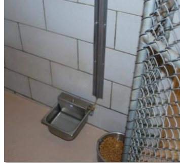
Supply lines for automatic waterers are vulnerable to damage from dogs. Photo above shows a guard that was installed over the copper pipe.
