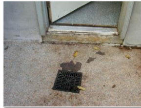
Old and chipped resinous floor
