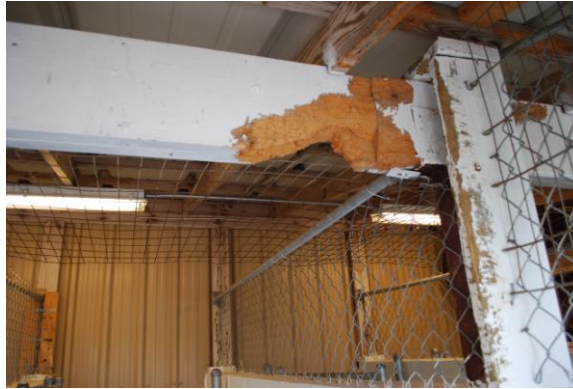
Damage was caused by a pit bull dog.
