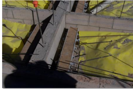
Photo above shows incorrect installation. Steel is uneven and vapor barrier is not taped.
