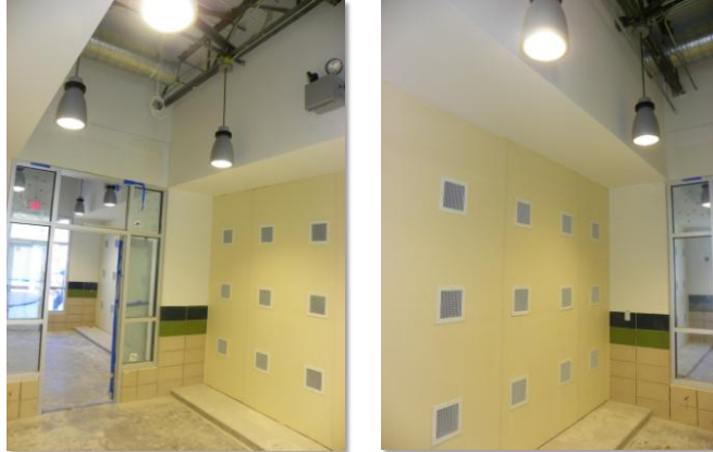
Photos shows the ventilation system behind where the bank of cat cages will be installed.
