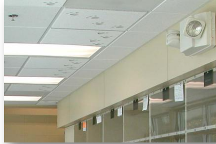
Paw print, acoustic lay-in ceiling system
