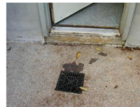
Old and chipped resinous floor
